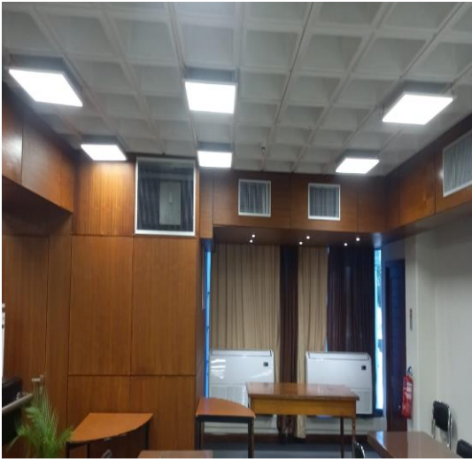
Fig 11: Indoor Air-conditioning System
