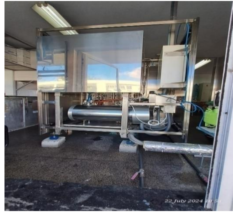
Fig 8: In-built Steam Boiler
