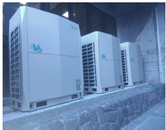
Fig 10: Outdoor Air-conditioning system
