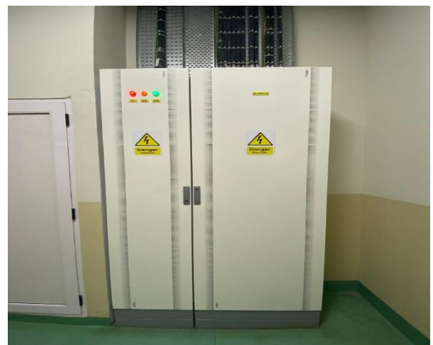
Fig 2: New Main Distribution Board
