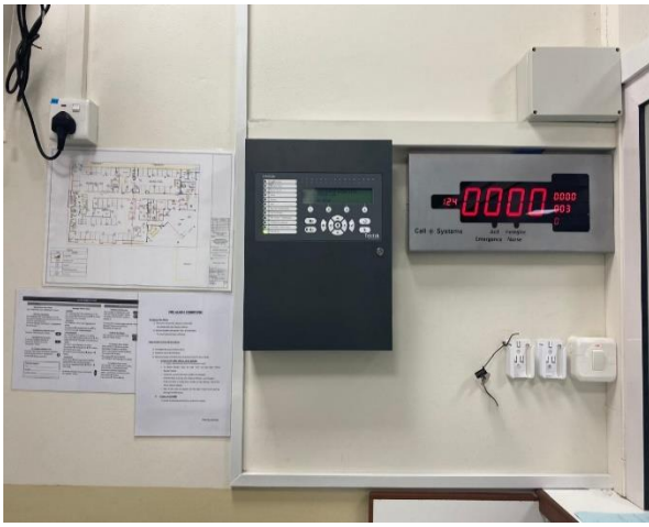
Fig 3: Fire Alarm Panel
