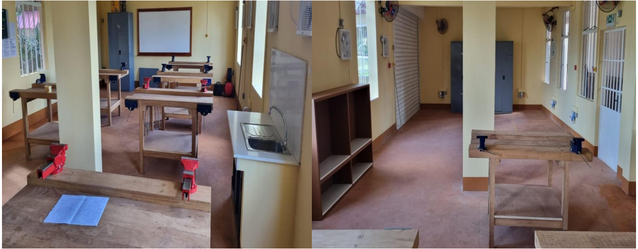
Conversion of existing classrooms into DC/DT workshop with furniture and drawing room.
