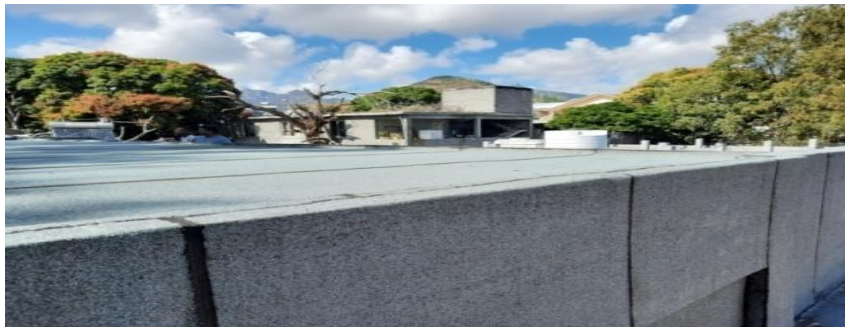
Waterproofing Works at St Croix Methadone Centre and Waterproofing Works at Dr F.Bouloux AHC
