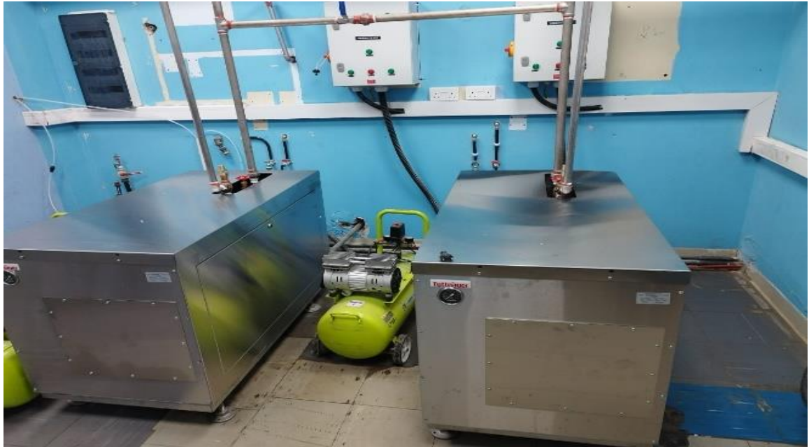
Steam generator, external boiler and control panel for Autoclaves 1 & 2
